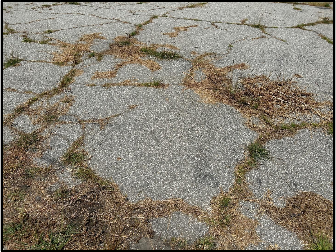
Figure 4.3-3 CLOSEUP OF PAVED SURFACE WITH FISSURES AND VOLUNTEER VEGETATION
